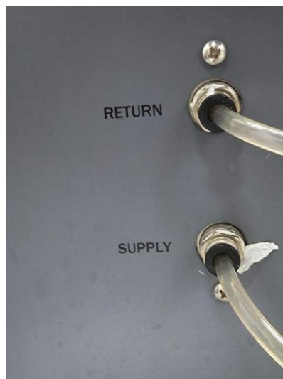
Figure 4-7 Cooling water circulator end water pipe connector
